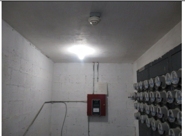
Smoke Detector and Alarm Panel
